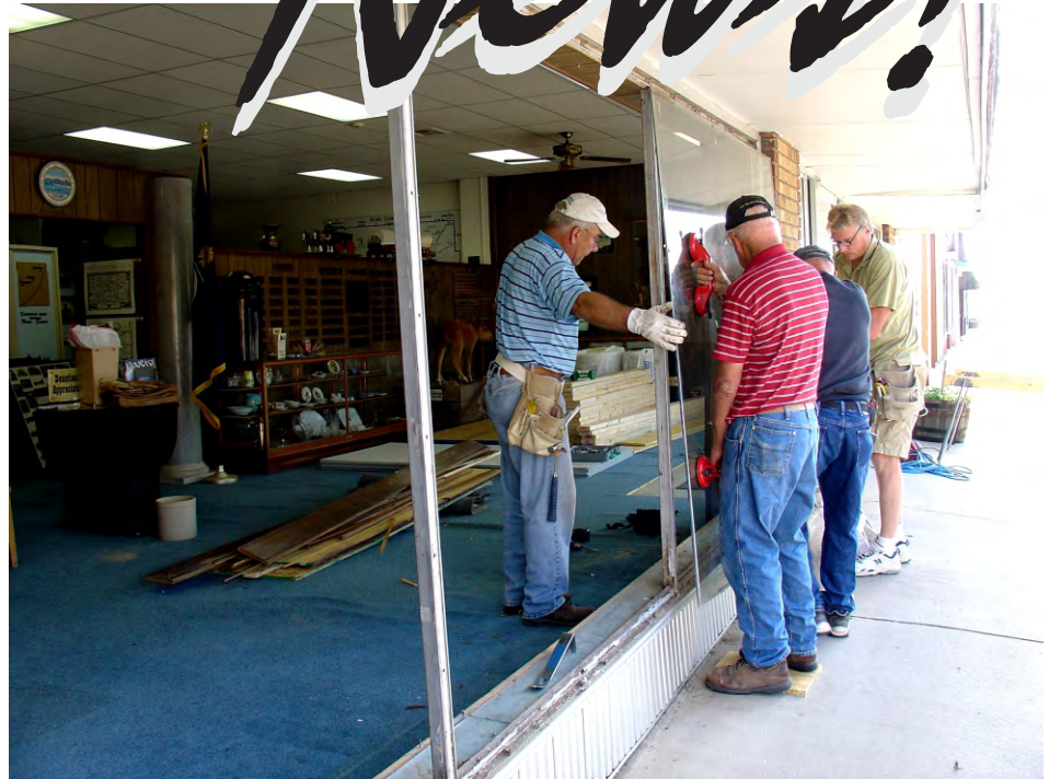
Carpenters Ken Isaac and Barry Friesen work with Ralph Classen and Glen Feldman to remove the glass. The glass was used by Ralph and Glen to replace broken windows in their buildings down the street.
